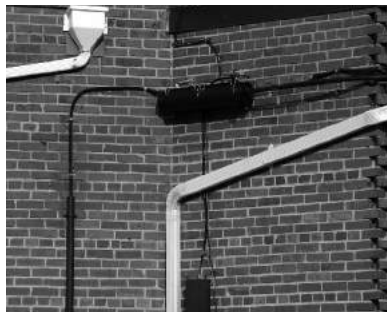
Downspouts – the wrong way! Note also the improperly located utility feeds.
