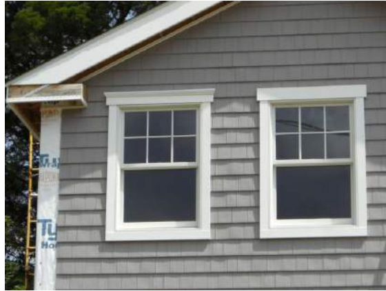
Trim with proper proportioning – 4" for windows, 6" for corners. Crown mould has been put on one of the windows.
