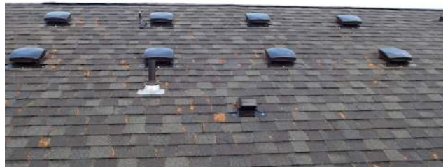
Roof vents – the wrong way!
